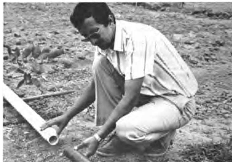
Mounting an alternative ditch irrigation system for a bean crop, suitable for small parcels. The work is being carried out under the Jipijapa Integrated Rural Development Program.
