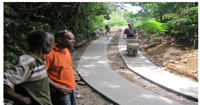
IICA Technical Specialist and FAO Correspondent inspect one of the rehabilitated farm access roads
