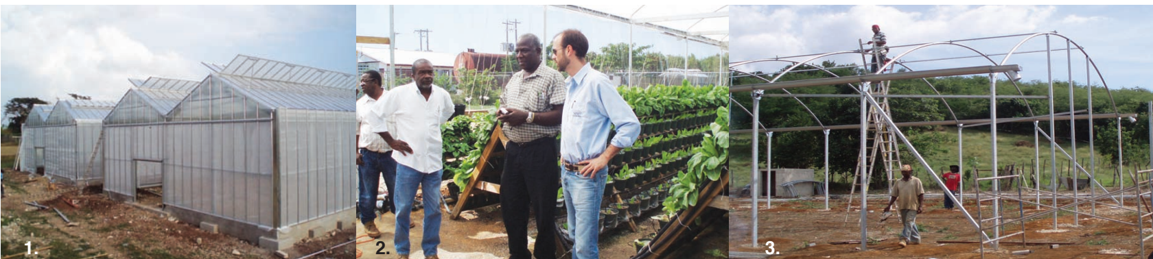
(L-R:) 1. Four mini research greenhouses completed. 2. Representatives of MSC Invernados meet with JGGA members and visit local greenhouses before completing the new standard greenhouse design. 3. The first of the newly designed greenhouses under construction in St. Elizabeth.
