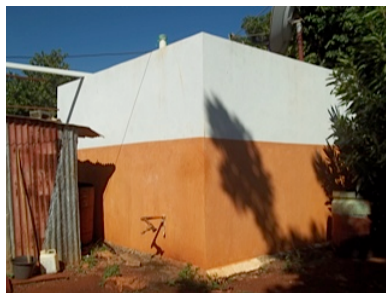
Figure 2: Rainwater Harvesting Tank - Comma Pen, St. Elizabeth
