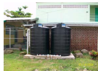
Water harvesting tanks at the St. Patrick's Roman Catholic Church
